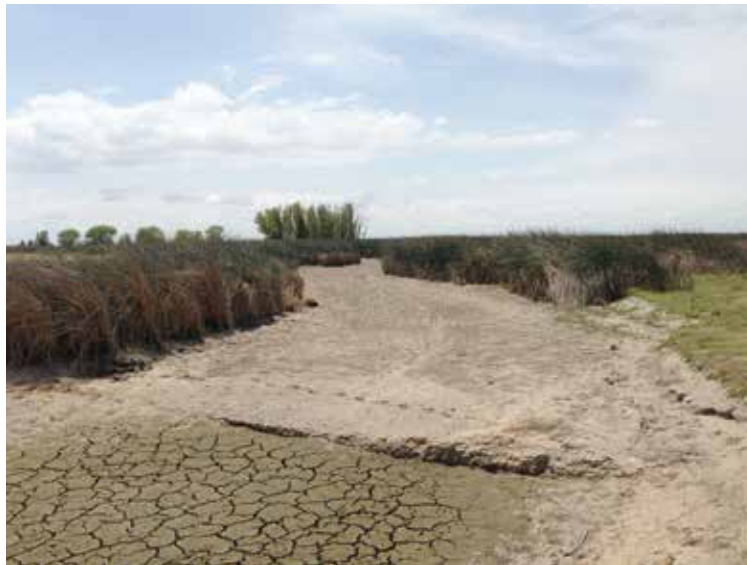
FIGURE 3 Channel renovation project on BKS North Course, Phase #3. Conservancy efforts to keep marsh complexes fully functional continued in 2013. The top photo shows a “before” channel on Pond Q on the BKS North Course. Note how the channel had filled in from eutrophication, particulates settling out, fossorial animals’ work, etc. The photo below shows the same general area but after channel clearing had taken place. See how tule has been preserved so as to minimize disturbance and allow for Giant Garter Snake re-entry and re-colonization after re-flood. (Conservancy staff photos.)
