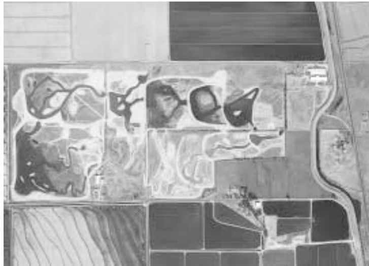
BKS Restoration and Enhancement construction project, Summer 2001. Aerial photo of the Conservancy's BKS reserve in North Sacramento County showing construction underway. The project represented the Conservancy's first restoration and enhancement effort. Photo: CalAero for The Natomas Basin Conservancy.
