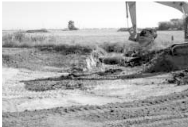
Water Cutover on Betts-Kismat-Silva Restoration and Enhancement Project. The Conservancy began work to construct managed marsh on the 338-acre BKS preserve in North Sacramento County during 2001. Photo depicts the first water to flood up managed marsh on the site. Photo: The Natomas Basin Conservancy.
